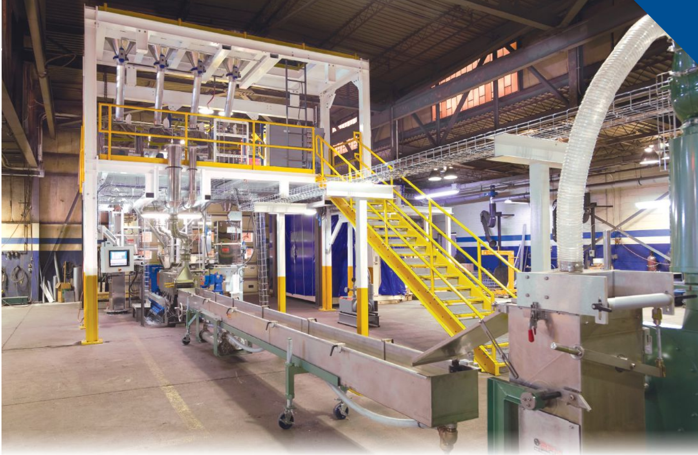
Figure 2: A compounding control center houses the extrusion system's electrical and control infrastructure, including an Allen-Bradley CompactLogix programmable logic controller (PLC), Allen-Bradley PowerFlex 755 ac drives, and solid-state relays from Rockwell Automation. A separate utility control center houses the system's utilities and information server.
